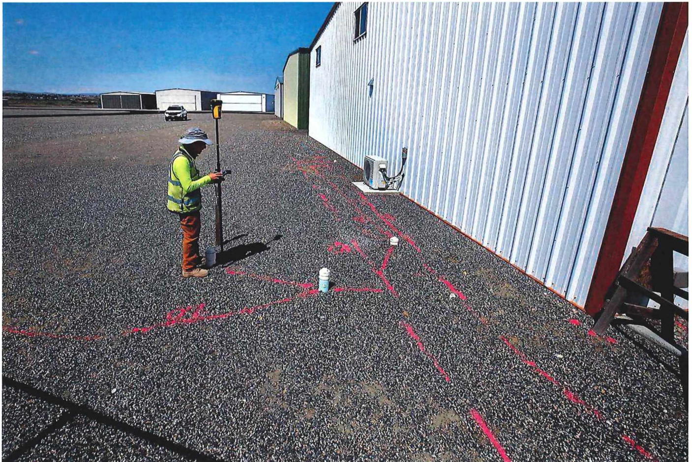
Mark Villa, of Geophysical Survey in Kennewick, maps out underground lines he marked with paint by using ground penetrating radar inside the fenced hangar area at the Port of Benton's Richland Airport. Bob Brawdy bbrawdy@tricityherald.com
